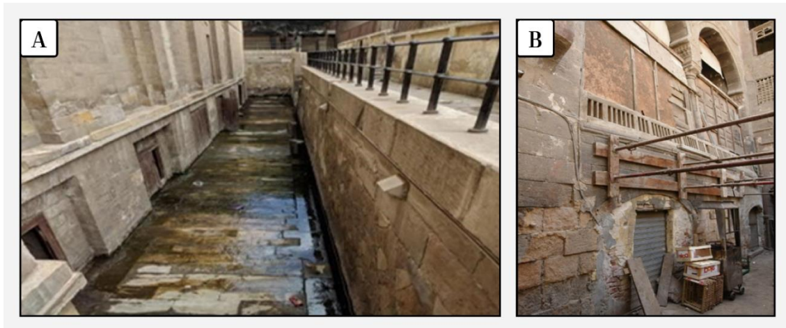
Fig.11. A) The problem of rising ground water level in Al-Saleh Tala'i Mosque; B) Al-Alili's house was not evacuated despite a decision to evacuate it.
